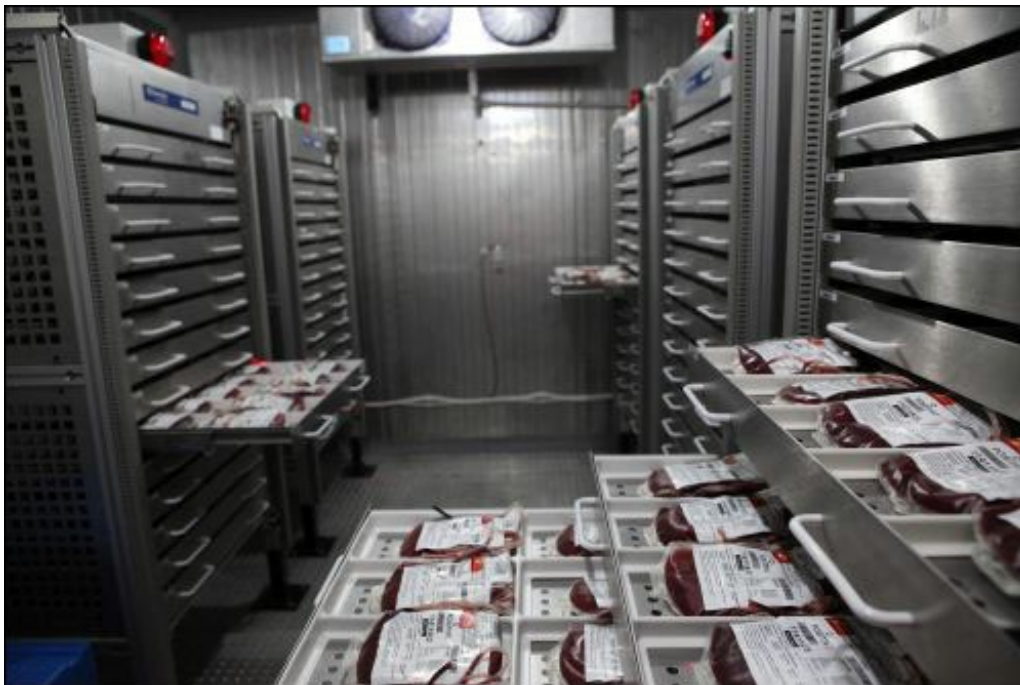
At the state blood transfusion center's cold storage room, five blood storage racks have been fitted with RFID readers and antennas.
