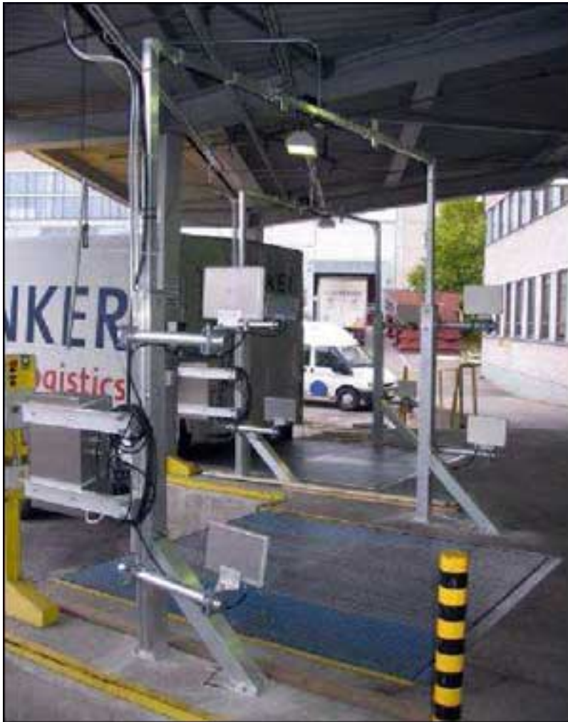
RFID readers installed at ABB's loading platforms are used to verify that the correct products are loaded onto trucks.
