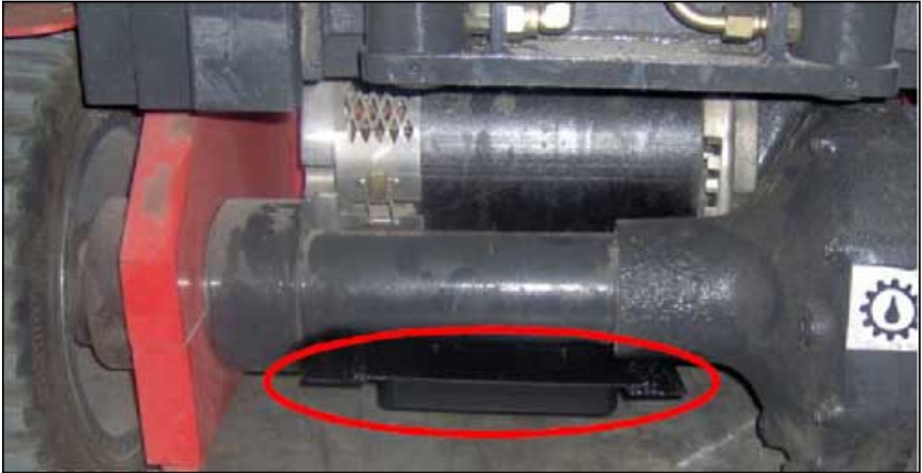
At its warehouses, Tetas installed RFID interrogator antennas under its forklifts, in order to read location tags embedded in the floors.
