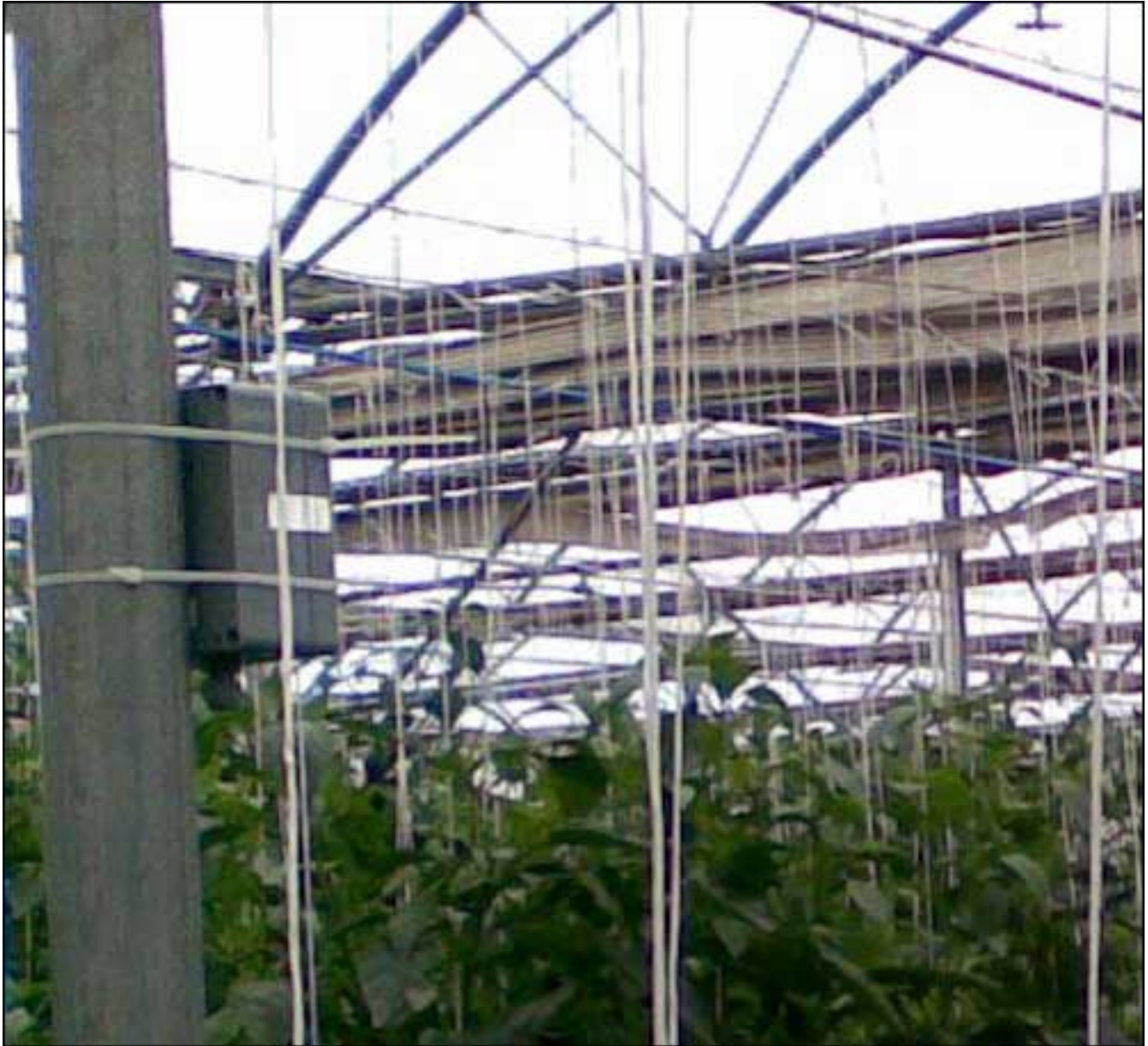
A ClimateMinder wireless sensor node (attached to a pole) measures environmental conditions at a greenhouse in Turkey.
