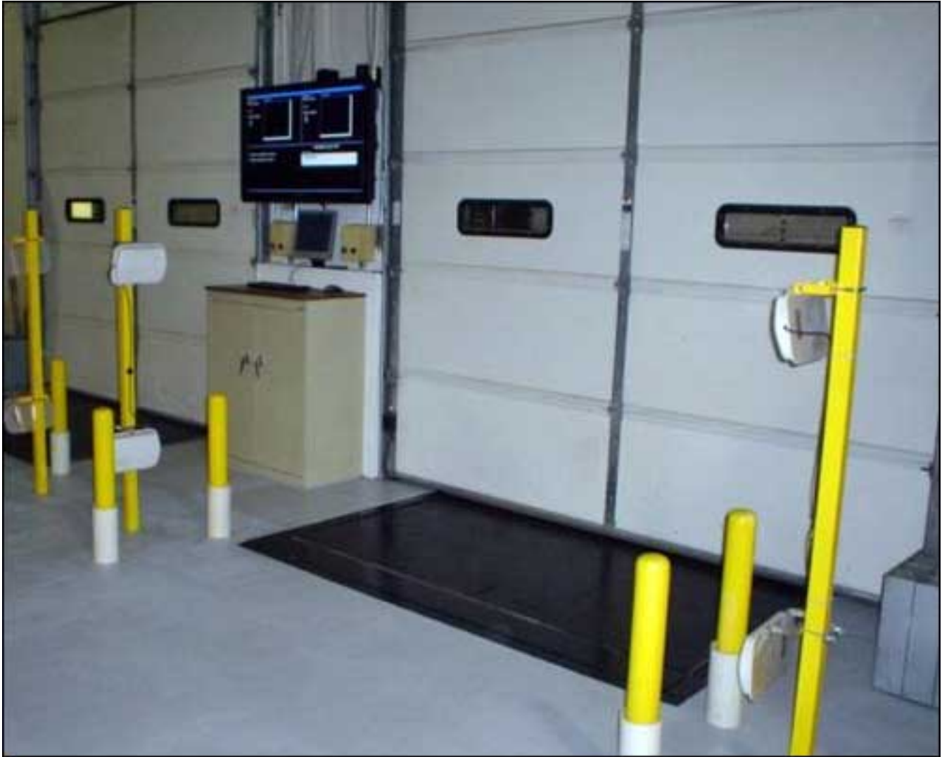
Color Point's RFID-enabled dock doors
