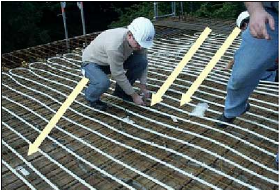
Temperature-sensing RFID tags were installed within the building's concrete ceiling.
